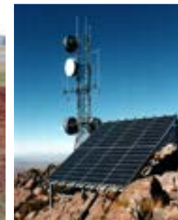
Utility microwave repeater network
