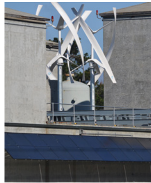
SES Hybrid solar and helical axis turbine wind power system for US Navy R&D.
