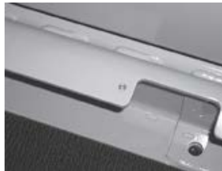
Figure 2: Adequate Paint Penetration
