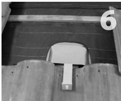
6 Proceed with weatherproofing using three-course method or lapped paper method.* When using paper method, cut a piece of underlayment 18" wide to slide under the course above and over the sub-flashing. If course above is too high, you must use additional underlayment to ensure proper overlapping.
