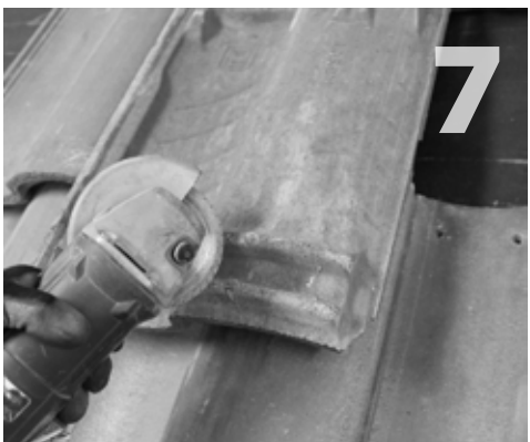
7 Replace the tile above the hook. If necessary, notch the bottom of the tile to make space for the raised hook.
